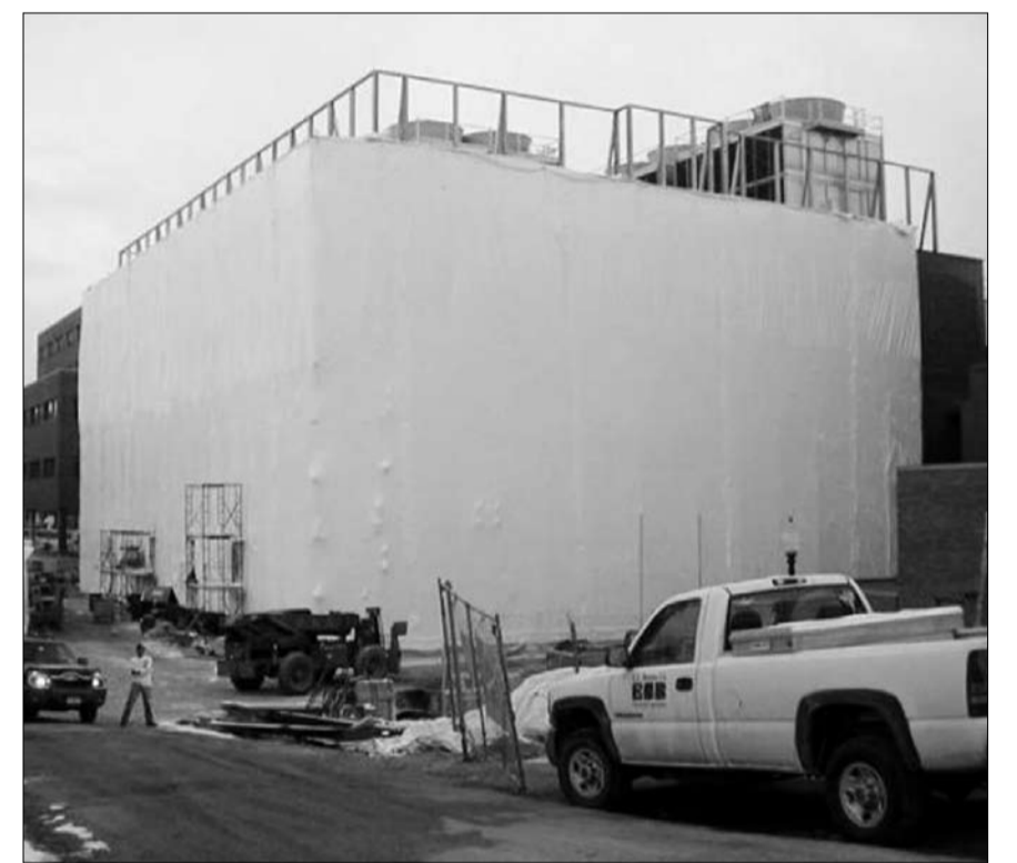
Companies are shrink-wrapping larger buildings as the construction industry leaves unfinished buildings and developers look to work year round. PHOTO COURTESY OF ZAP ENTERPRISES
